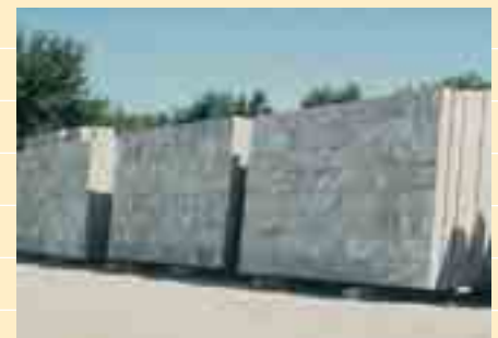
Architectural precast panels for the new wing of the Joslyn Art Museum, Omaha, Neb., are clad in Georgia marble to match the original stone building constructed in 1931. Labor and material cost were reduced using this system compared to traditional stone cladding systems. (Architect: Henningson, Durham & Richardson Inc.)
