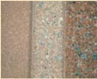
The single concrete mix shown here has three different finishes. From left to right, they are acid etch, sandblast and retarded. This multiple-finish technique offers an economical, yet effective, way to heighten aesthetic interest.
