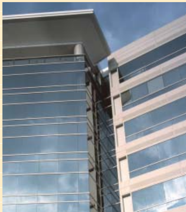
Detail of a glass to precast plane transition at the Waterway Plaza, The Woodlands, Texas. Note how the hue of the mix design complements the window frame coating. The precast panels were fabricated from a single mix containing white Portland cement, coarse aggregate (Texas Pink), and fine aggregates (Black Star, Big Sandy Sand, and White Sand). After casting, the panels they received light or medium sandblast texturing. Photo: courtesy of Gensler.
